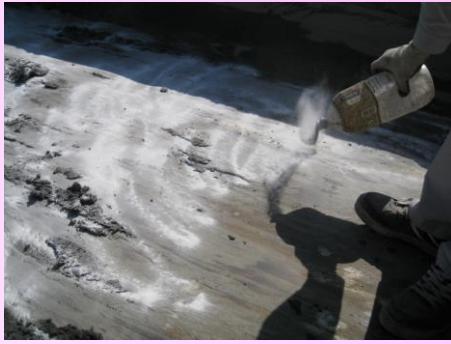
Apply an appropriate amount of Mud Suberu on bed of dump truck
